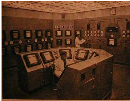
Fig. 2. — Control room of a British nuclear power plant.
